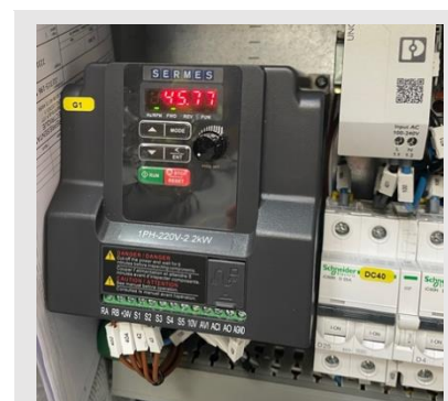
The Variable Frequency drive in the electric box.
